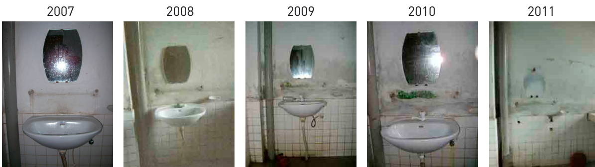
Going, going, gone...the demise of a basin in the only toilet in the outpatients department of the district hospital. (Central urban)
