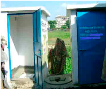
New public latrines have been installed in the north urban study area to replace these old ones but improper construction means they drain out into the nearby open space
