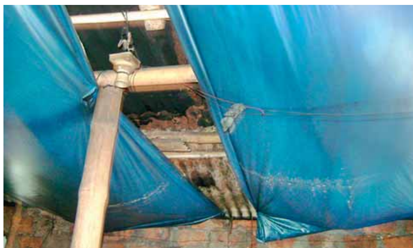
Ceiling repaired with polythene sheets to prevent rain water from coming in
