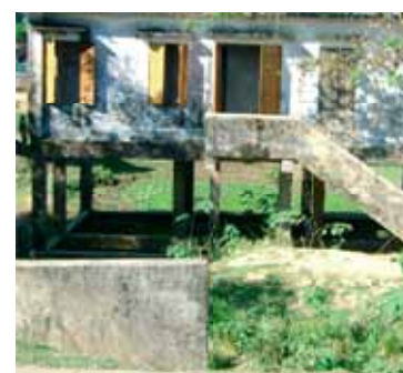
Poorly constructed and poorly maintained Community Clinic.
