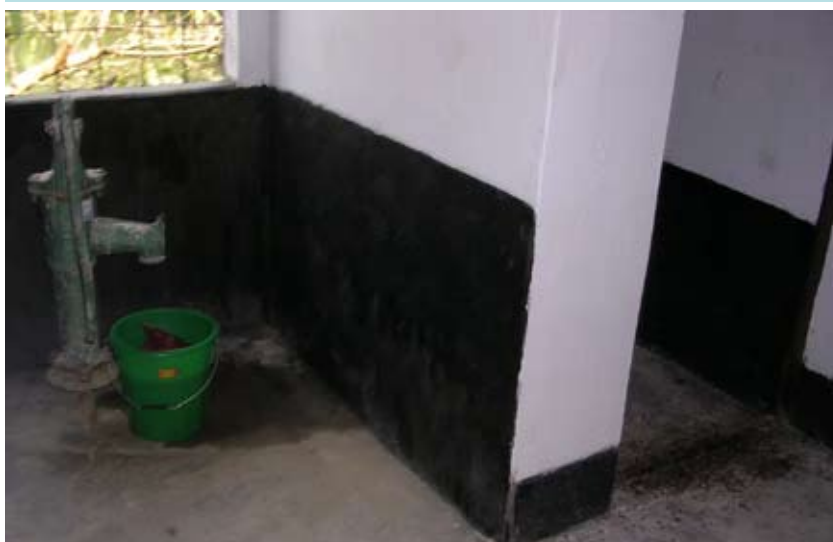
The tube-well at the newly opened Community Clinic is not working (Rural South)
